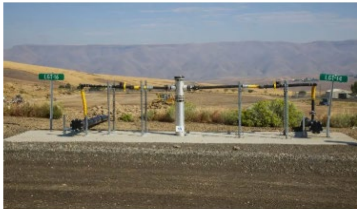
Figure 10 - LFG Monitoring Station
